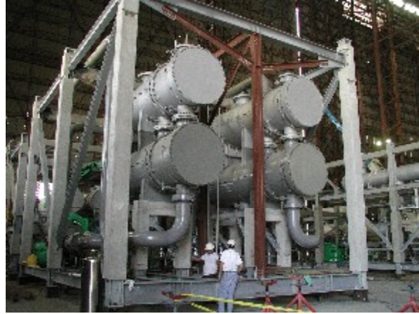
Figure 6-2 Example of exchangers being bundled on a module with valve manifolds located at the rear of the module. The lower frame of this module was buried in the concrete slab at site.
