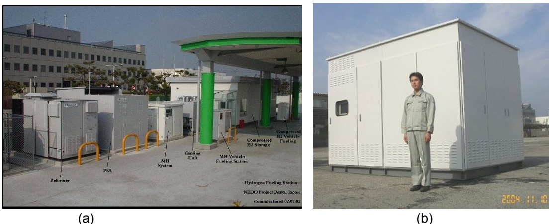
Figure 6 Osaka city hydrogen filling station using Osaka Gas reformer (a) Osaka Gas Compact reformer HYSERVE – 100 (100 Nm 3 ).
