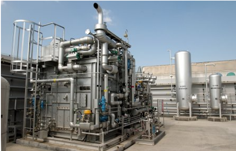
Figure 7 Mitsubishi Kakoki Kaisha naphtha reformers (a small 50 Nm 3 /h type is installed in Yokohama Asahi hydrogen station)
