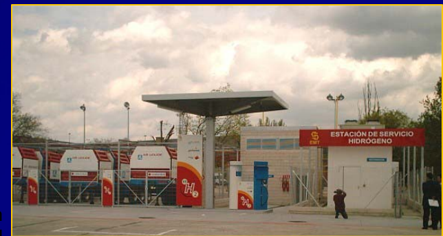
NG reformer station Madrid
