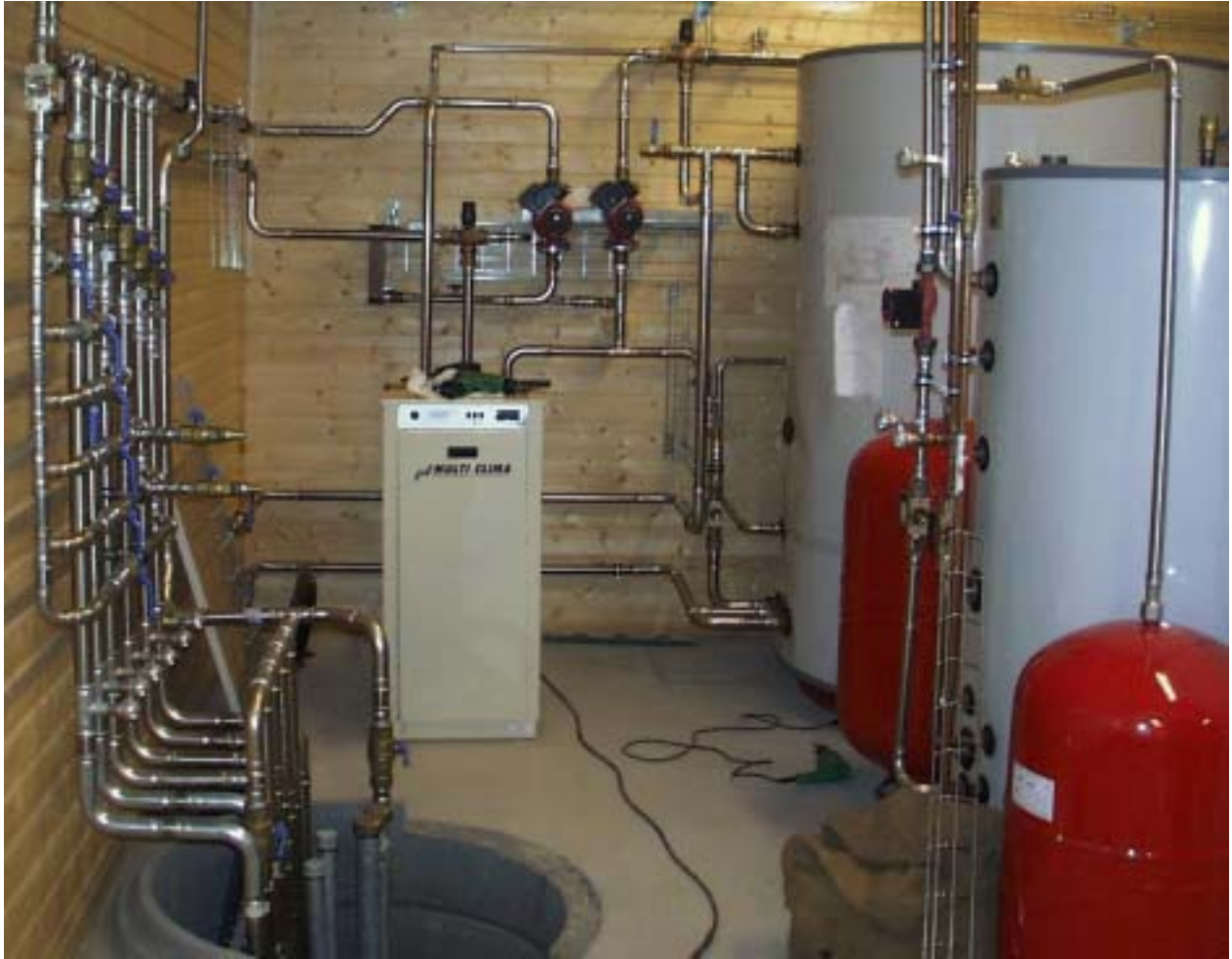
Figure 6: A view of the storage tank and the piping inside the thermal cottage
