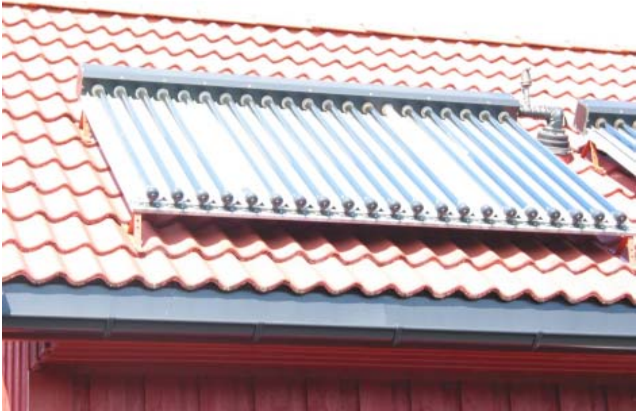
Figure 7: Solar collectors on the roof
